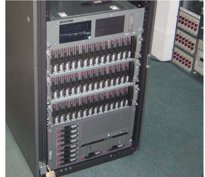
Server shown here with its initial 7.4TB start-up configuration.
